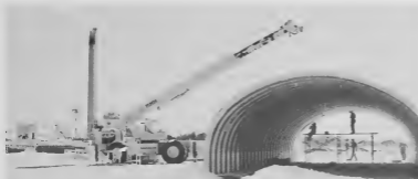
This Grove crane with a 35-ton lifting capacity, equipped with a telescope boom, here assists in erecting the Paint Shop, a steel prefabricated quonset hut.
